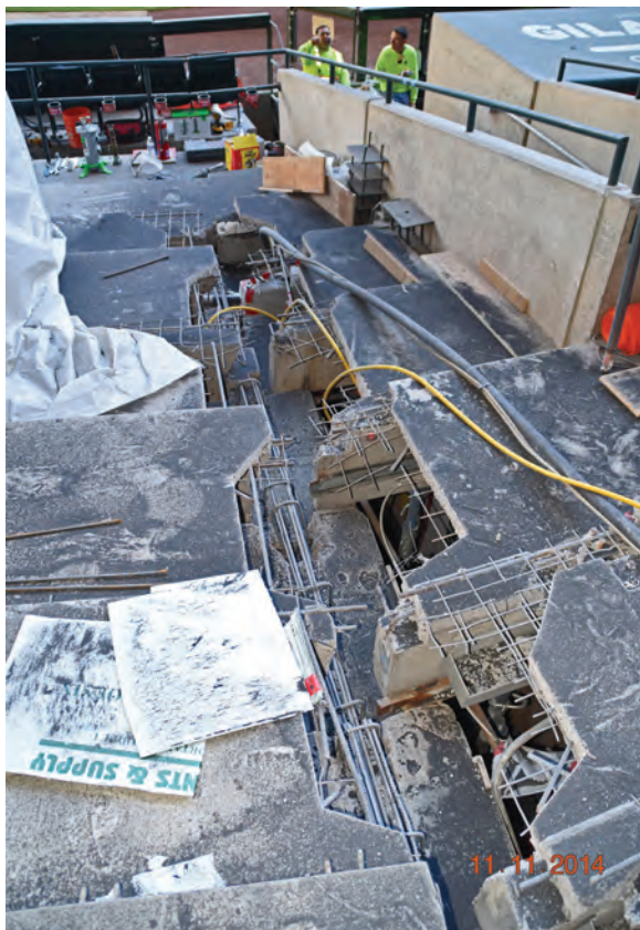
Fig. 7: Precast joint repairs—typical example of demolition required to repair the joints between the precast seating sections. Seismic restraint plates have been completely removed for replacement. Bearing repairs for stems have not started. Nearly every row was affected.
