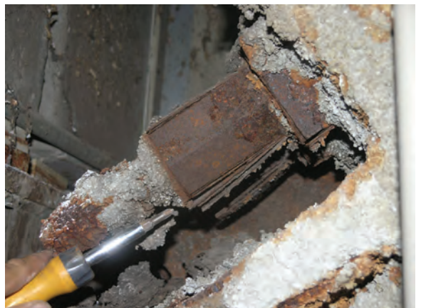
Fig. 4: Threaded rebar anchor nut—Severe deterioration of the nut. Corrosion of the threaded anchor rod is not visible due to fireproofing and debris.
