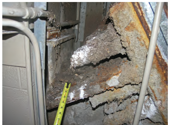
Fig. 5: Threaded rebar anchor—large mound at end of tape measure is peanut shells and debris washed through failed joint above.
