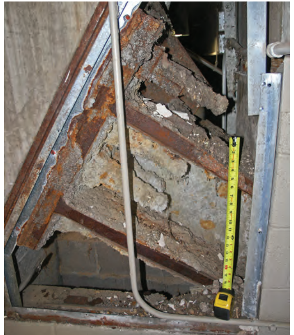
Fig. 3: Raker truss tieback anchor—connection between steel raker truss and concrete frame with sixteen 1-3/8" (35mm) diameter high strength threaded rebar anchor rods. Connection is completely hidden between two masonry walls in a dead space with leaking precast joint directly above. Spray-applied fireproofing absorbs water and never dries out.
