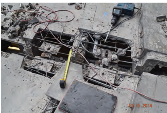
Fig. 8: Typical Precast Joint Repairs—Water leaking through building expansion joint between precast seating sections was absorbed by mineral wool fireproofing in the joint, resulting in severe deterioration. Large steel plates are seismic restraints.
