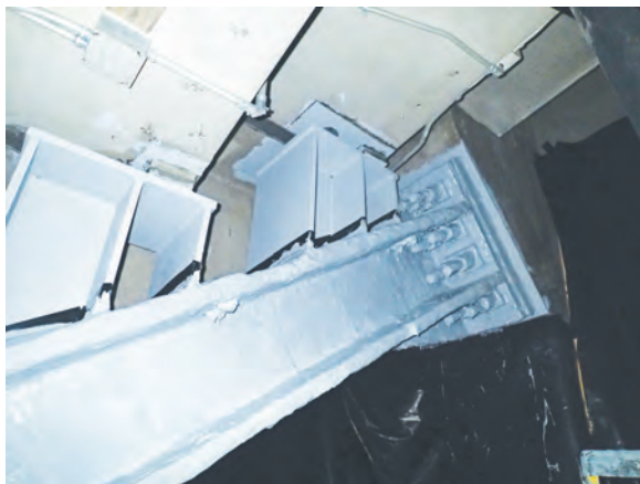
Fig. 6: Raker truss tieback anchor connection—completed repair with epoxy intumescent fireproofing to achieve 3-hour fire rating and provide corrosion protection to the beam and threaded rebar anchors.
