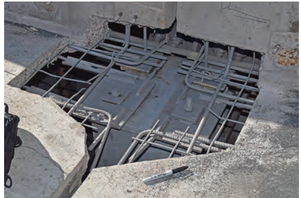
Fig. 9: Typical precast joint repairs—seismic restraint plate (embed with bolt) and precast bearing seat assembly (below prestressing strands) after existing plates replaced, rebar welded back, and sandblasted prior to epoxy coating and pour back.
