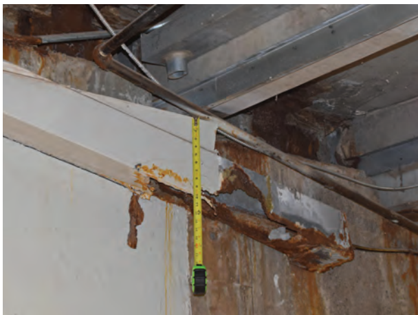
Fig. 2: Bottom side of seating riser at support—seating riser bearings and seismic restraint plates are visible on the bottom side. Moisture penetration through building expansion joint into mineral wool (each side of L-shaped plate) resulted in severe corrosion. Rain gutter system completely corroded through as it enters uninhabited space.
